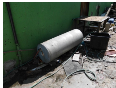
A typical hot water installation ☹
