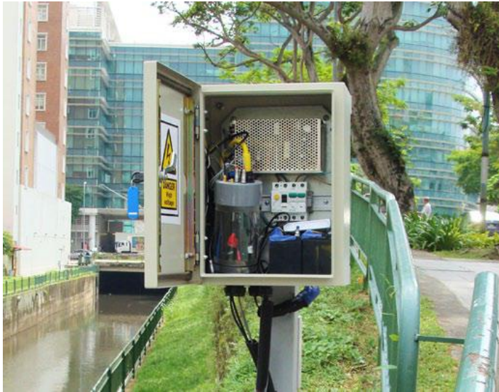
Figure 39 - A Sensor panel in the CBD area of Singapore.
