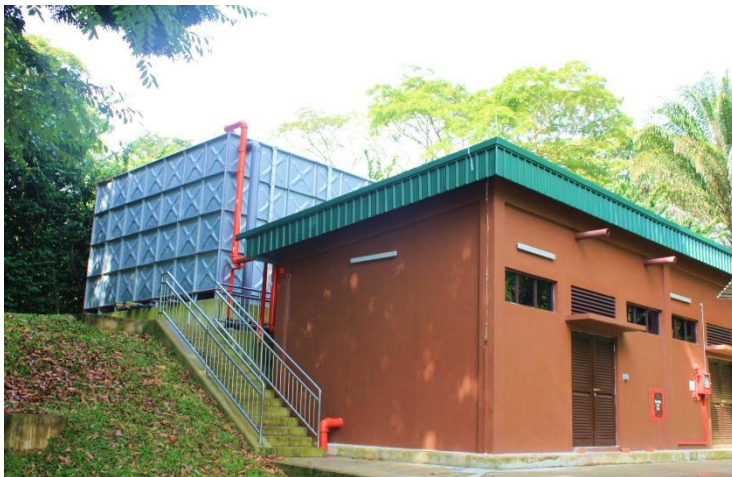
Figure 34 - The Pump Room and water tanks for fire and washing supply.
