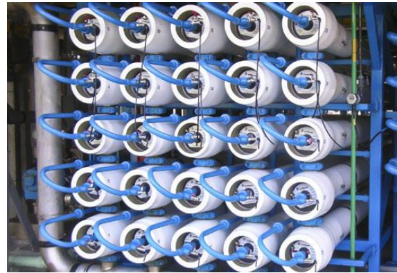
Figure 77 - Water processing at the VSP entails the passage of microfiltered water through a series of RO Membranes.
