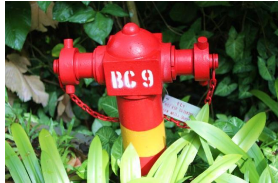
Figure 37 - A Fire Hydrant in the Zoo premises, the tag on the side states "Not for Drinking, Raw Water Supply"
