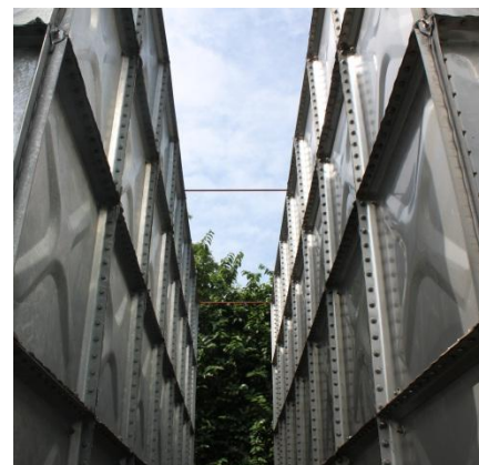
Figure 35 - The GI Tank of left and Stainless Steel Tank on Right.
