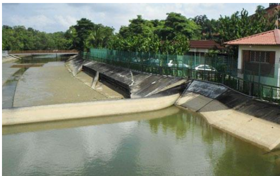
Figure 76- Inflatable rubber weir traps rainwater, which is processed via the VSP's brackish water workflow.
