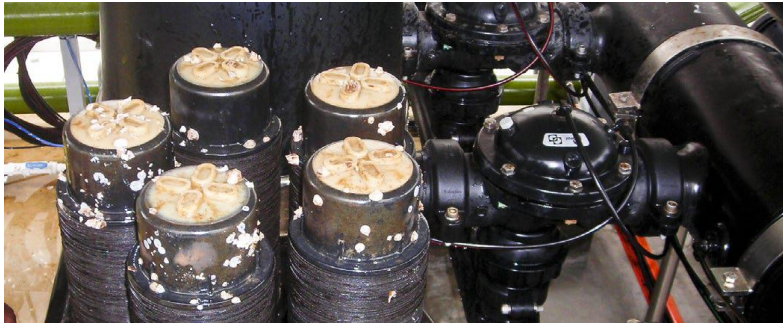
Figure 78 - VPS Pipelines overgrown with barnacles and mussels.
