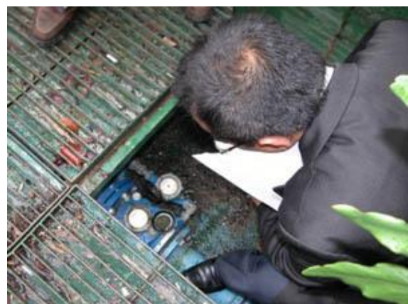
Figure 27 - Regular monitoring of water consumption.
