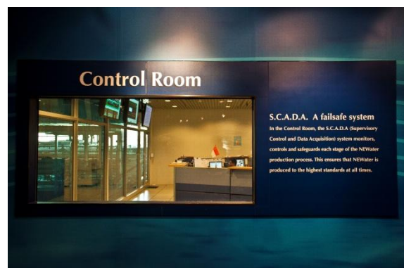
Figure 69 - The NEWater Control Room deploying SCADA assures round the clock monitoring.
