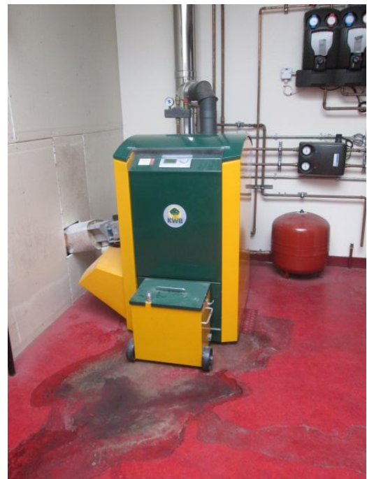
Bio mass boiler – Cork CIT
