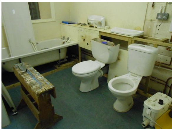
Fixture installation and connection area
