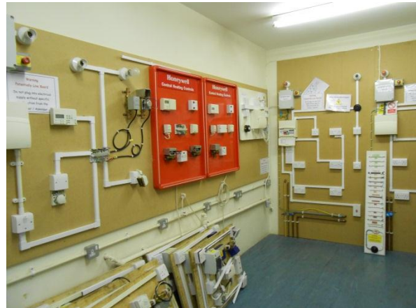
Electrical training room
